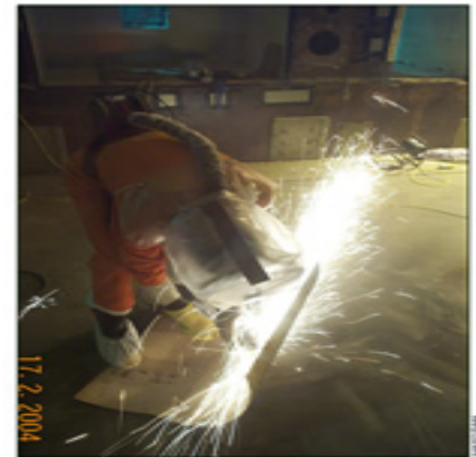
Size reduction of a floor storage bulk liner in the South Coast Line (WRS, 4.26.15.2)
